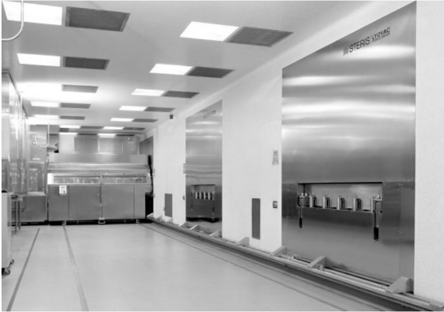
Fig. 2.73.3. Automated guided vehicle (AGV) running in a sterile corridor for the automatic loading and unloading of three freeze dryers. (Glaxo SmithKline, Parma, Italy).
